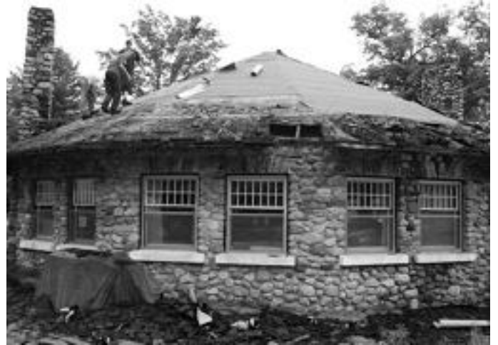
Work started on the Bigwin Tea Room in late September. Photo by Andy & Dorothy Barnet
